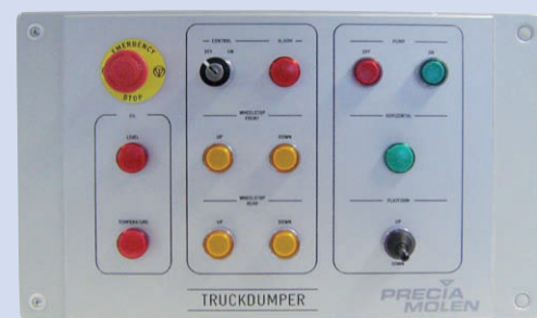
Detail of control panel for operation of the truck dumper
